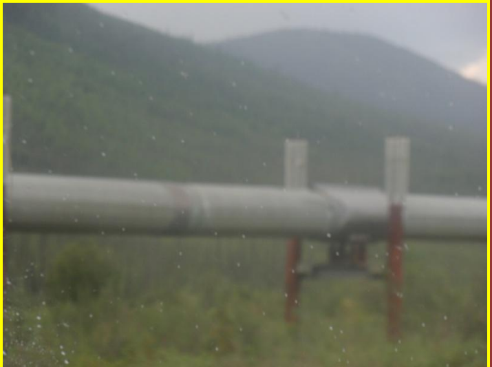
The pipe is not attached to the stands.
